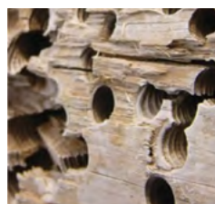
CARPENTER BEE DAMAGE
