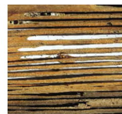
CARPENTER ANT DAMAGE
